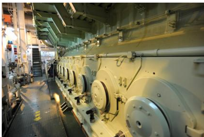
Alternate view of engine room
