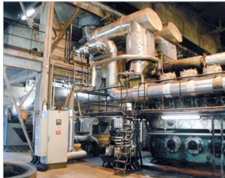
Figure 11: Power plant, Corsica
